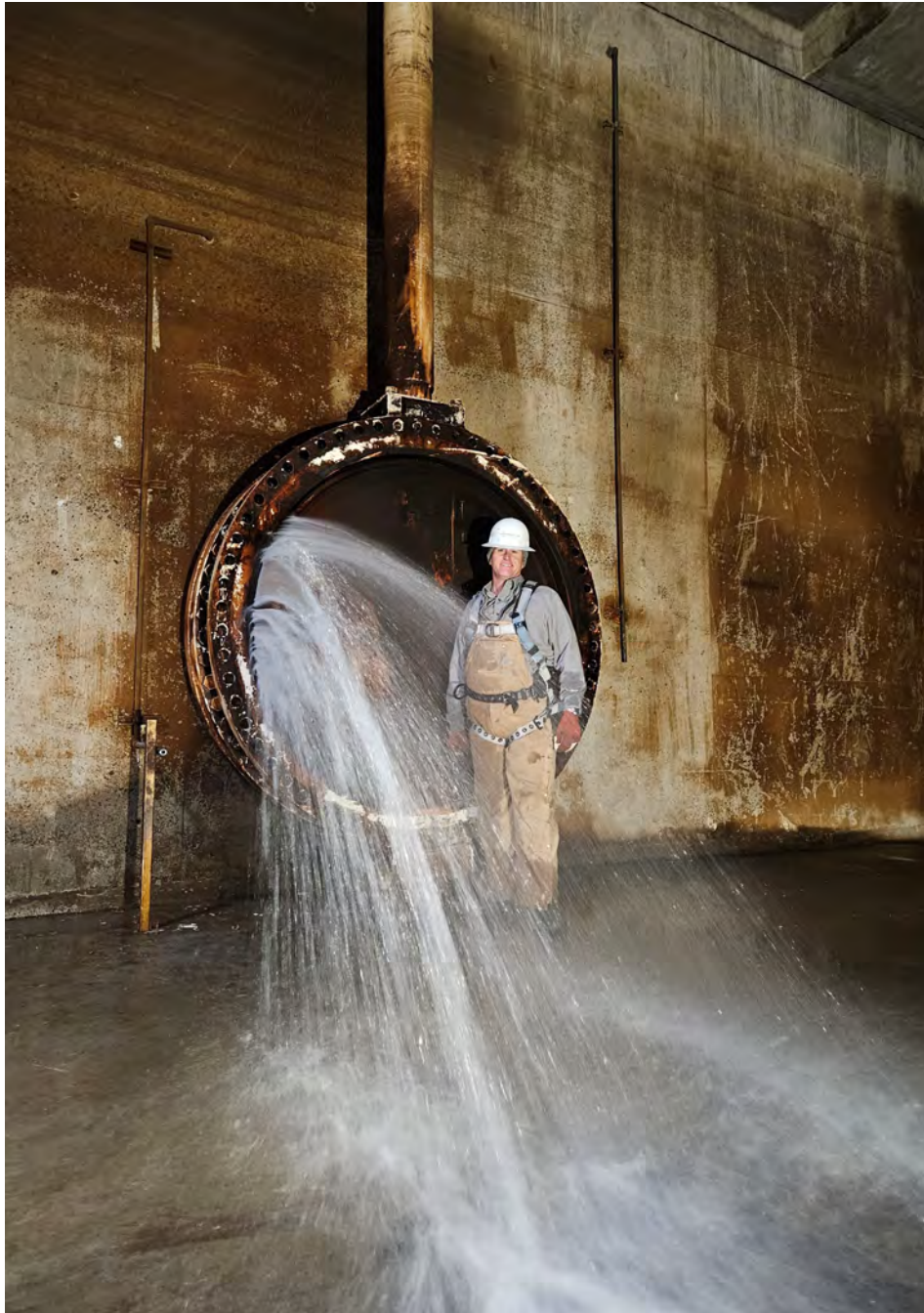
Photo: Chalk Bluff Clearwell Walkthrough before Disinfection Photo By: Craig Moyle, Water Equipment Specialist
