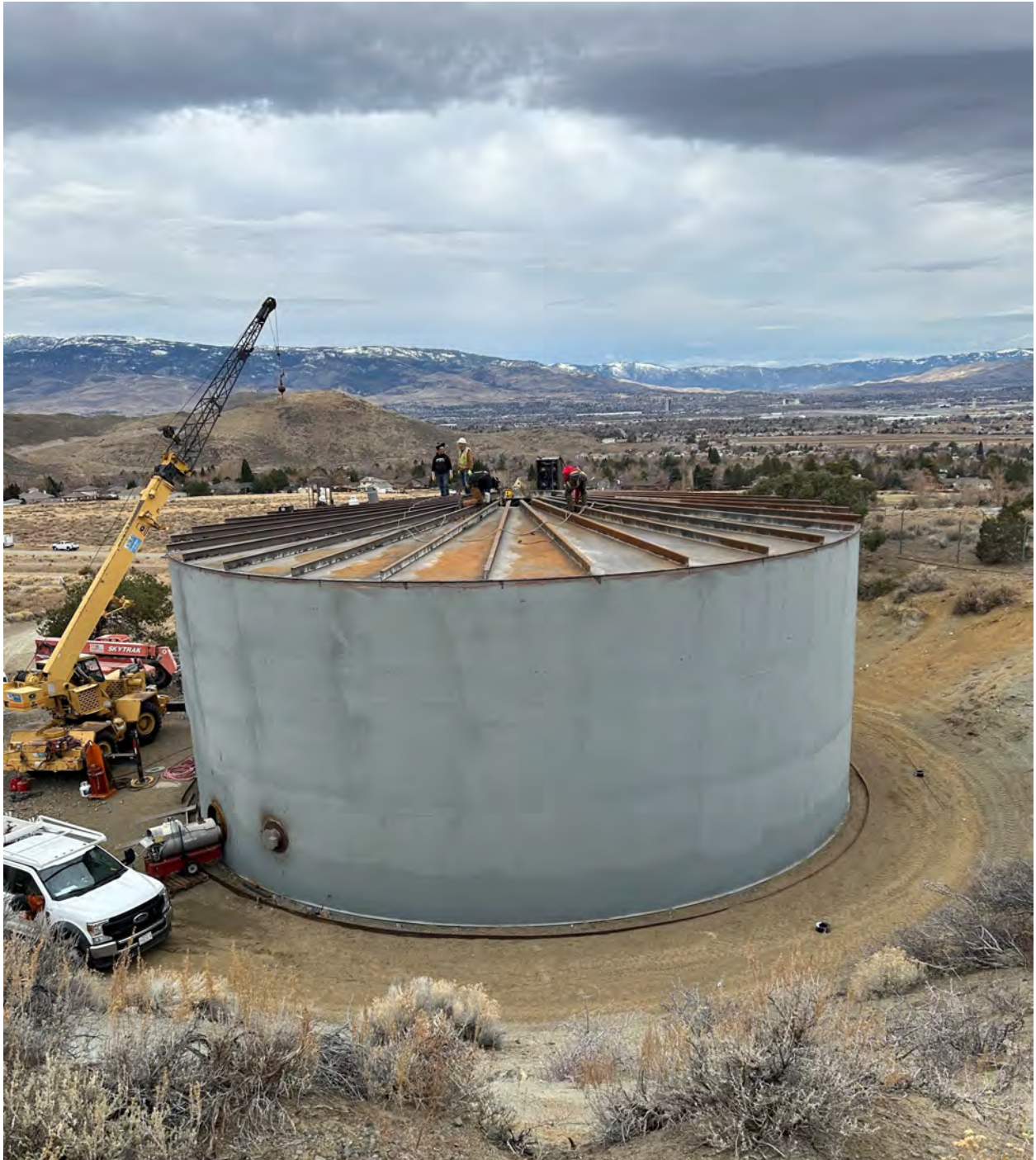
Photo: Hidden Valley Tank #2 Rebuild Photo By: Tarra Mora, Student Employee Engineering
